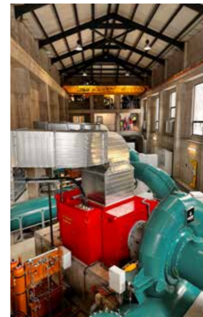
The massive engine room of the Akhalkalaki Hydropower Station
